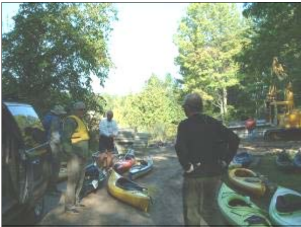
Hmmm... so where's the ramp? Piles of concrete presented a barrier to Newcomer paddlers waiting to launch on the Torch River, but helpful DNR workers got busy and created a temporary access for the group.
